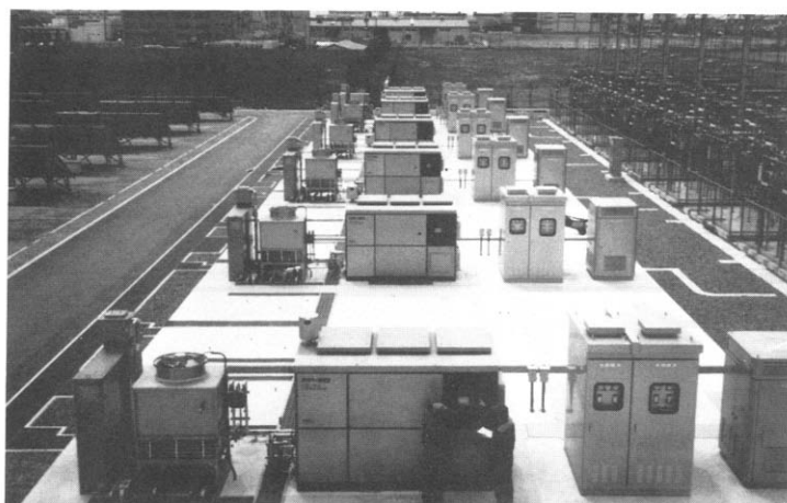
Fig. 4. General view of 50 kW PAFC plants at Rokko Testing Station (near Osaka).
