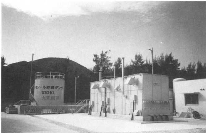
Fig. 9. General view of 200 kW methanol reforming PAFC plants installed on detached island.
